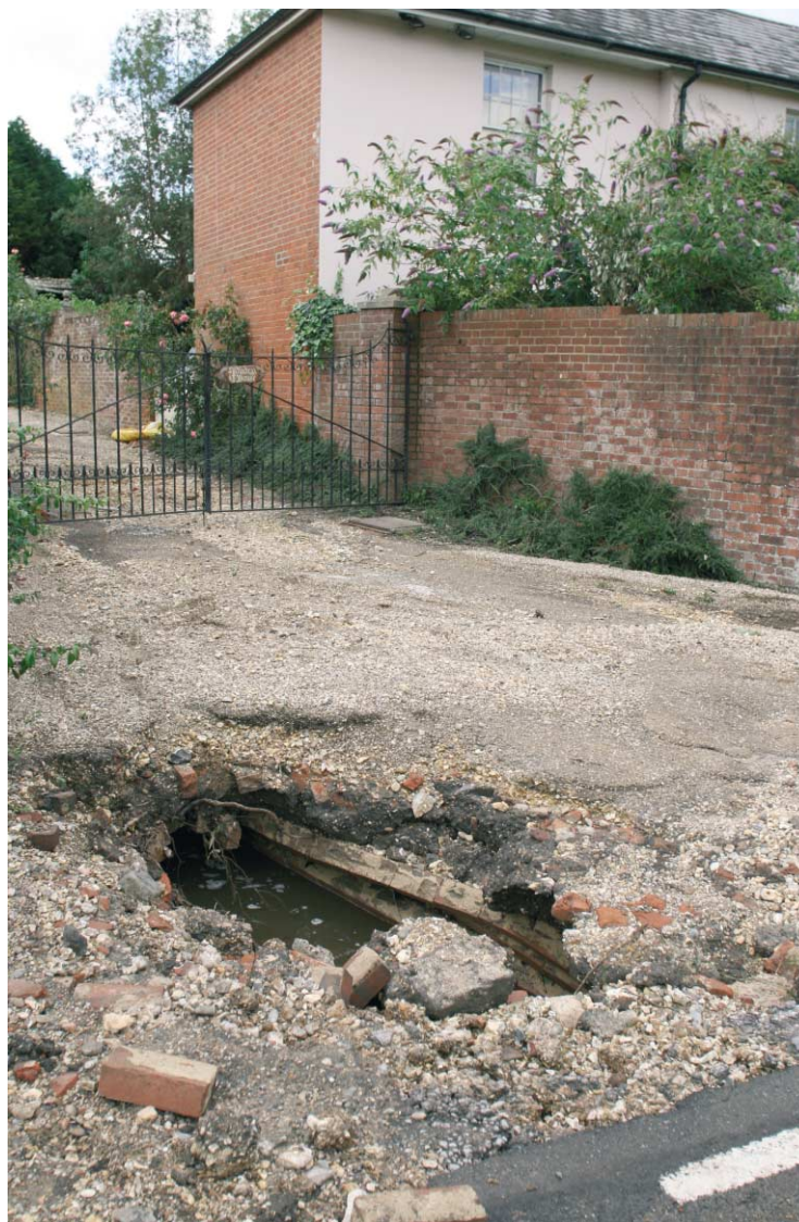
Figure 3. Damage to culvert in The Street, Stratfield Mortimer, as a result of the 20 July 2007 storm. National Grid Reference SU (41) 671 642. (Photograph © Stephen Burt.)
